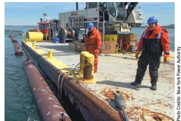
Photo Credits: New York Power Authority
