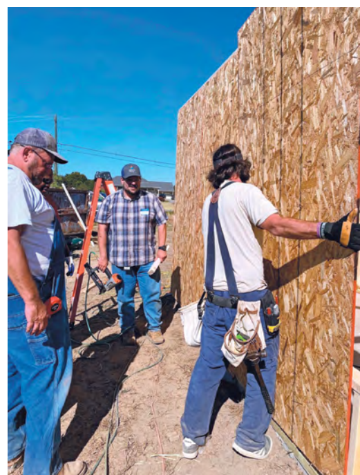
IBEW members volunteered with Habitat for Humanity and Alabama Power to build a new home in just 10 days for a family in need.
